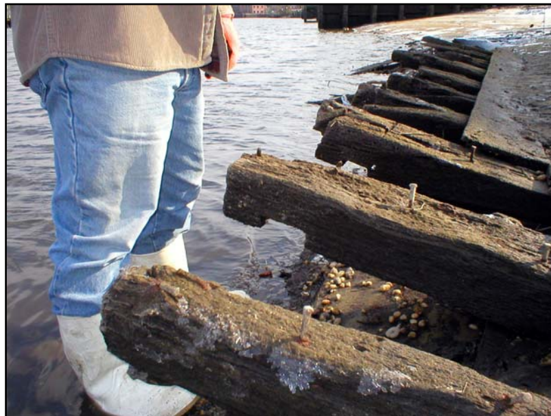
Frames showing limber holes.
