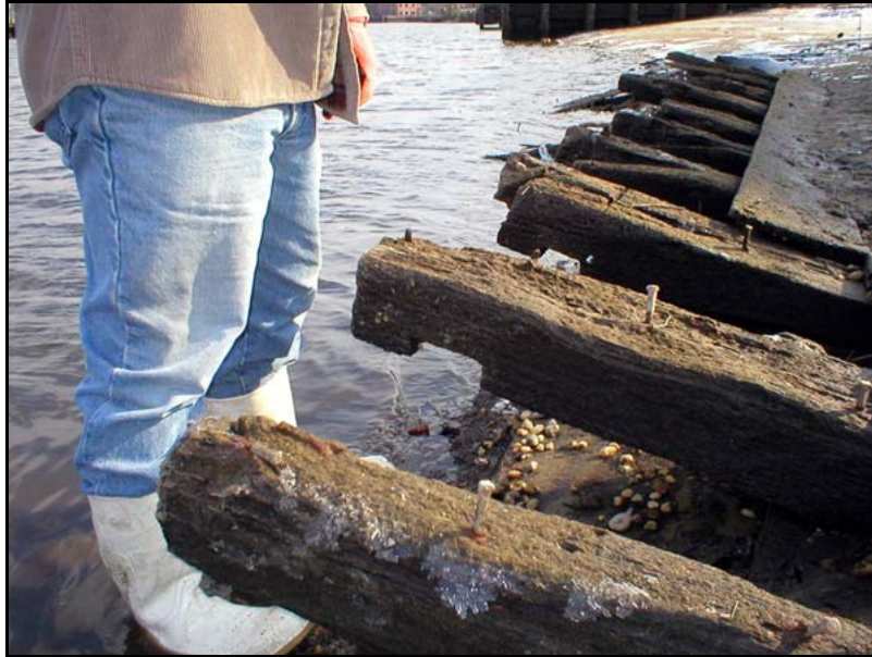
Figure 8. Site 18WC185, limber holes in frames.
