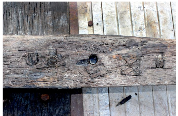
Timber with markings thought to be construction guides. Photo courtesy of MDOT SHA.
