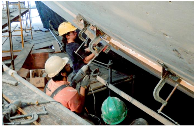
G. Steiner, R. Roa and R. Szimanski move a plank into position before securing it with lag bolts. Photo by J. Smailes.
