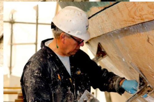
Above: C. Rowsom installs rolled cotton in the lower joint between the new planking and the original white oak planking from 1854. Below: J. Smailes removes excess glue from the top of a plank. Photos by D. Ehlers.
