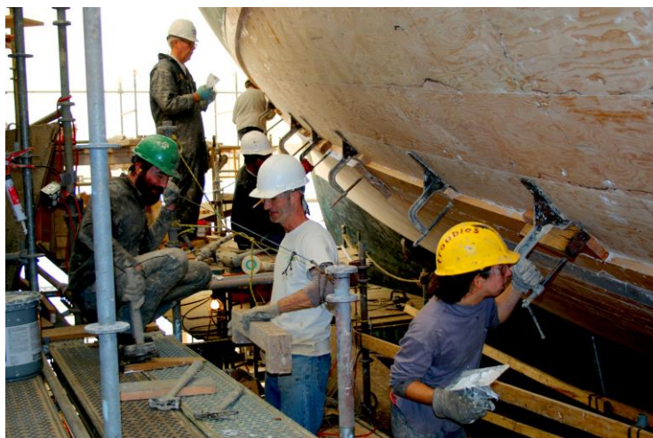
The planking team has just finished installing a plank. Next they will move the clamps and dry fit the next plank to prepare it for installation. Photo by D. Ehlers.
