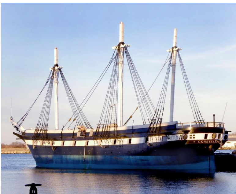
USS Constellation, out of drydock following renovations at the Curtis Bay Coast Guard Station in Baltimore, Maryland, and awaiting the tugs that will take her to her berth in the Inner Harbor. The upper masts had been removed in the fall and will be replaced later this year. Photo by J. Smailes.
