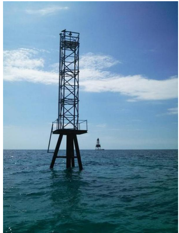
A new beacon has been erected to replace Carysfort Reef Light, shown in background.
