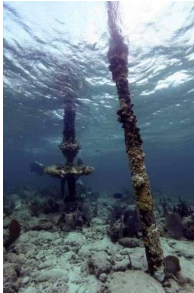
Totten Beacons: These navigation aids were placed on French Reef in the mid-1800s to warn mariners of the shallow structure that runs along the ocean side of the Florida Keys.
