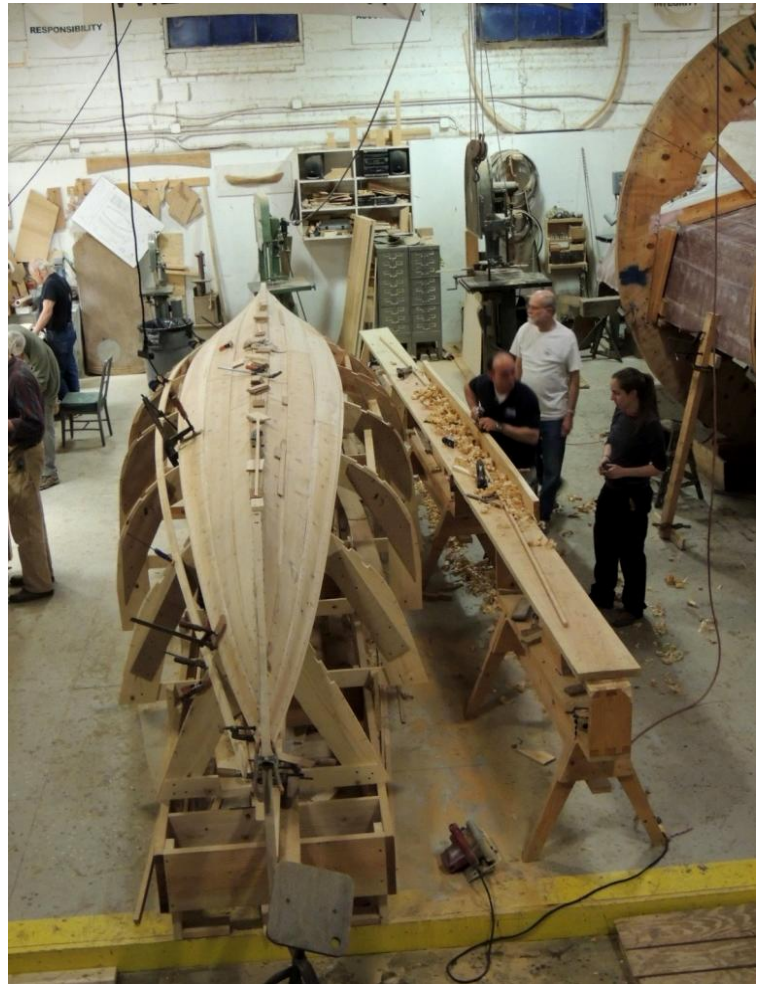
Planks are applied to the station molds, or forms, that bear the shape of the hull and guide construction. The planking bench, alongside the boat, is a convenient aid in shaping each plank before installation. The bench minimizes handling of materials during construction.
